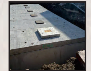
Under Ground Water Tank
